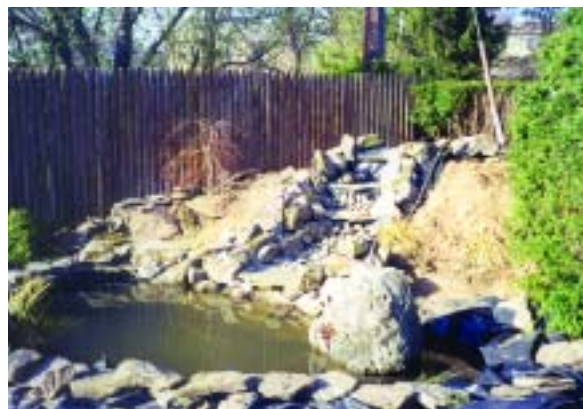
After excavating the soil for the pond, Brian could use the mound of dirt for carving in his waterfall.
