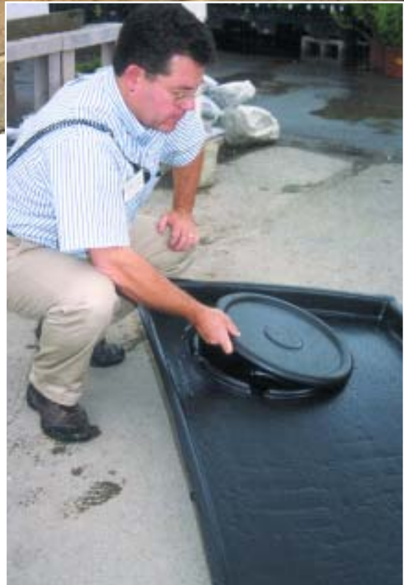
Place a small pump of 80 to 125 GPH in the sump area and fit the cover in place. Plug electrical cord into a GFCI-protected source, affix water tubing to your desired flowing feature, and arrange pebbles over the feature. Use coarse sand or small pebbles to create a bird bathing area.
