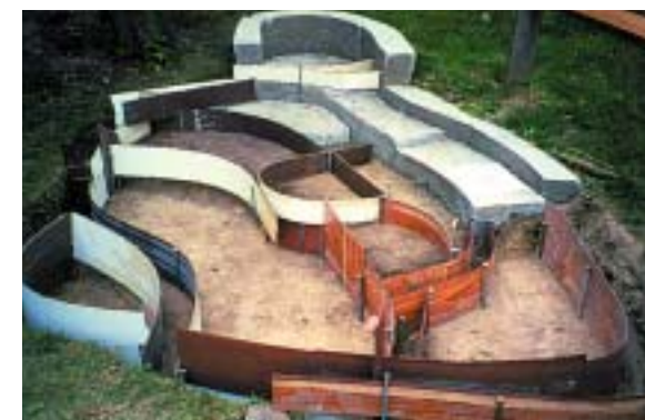
Flexible and thin wall panels were used to create forms for the concrete base.
