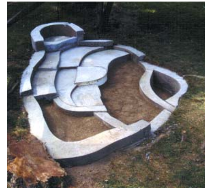
Concrete was mixed by the bag and filled into each section of the forms. The 12-inch railroad spikes holding the forms in place were pulled before the concrete had fully set.
