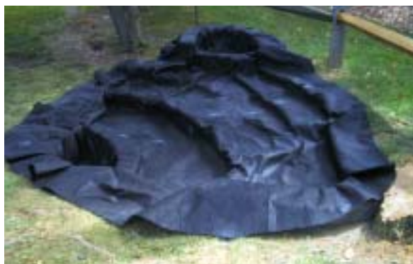
A geotextile fabric protects the liner for the long life of the pond construction.
