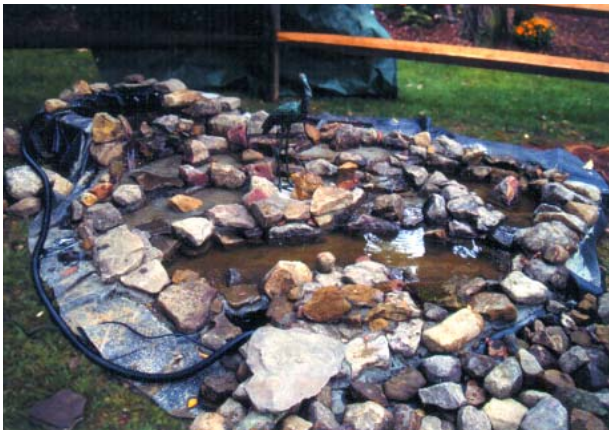
The plumbing from the submersible pump in the hidden reservoir would be buried to the entry point at the top of bird pond.
