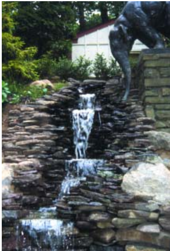
A large waterfall need not be made of large boulders. Every stone used in this construction can be managed by a single person!
