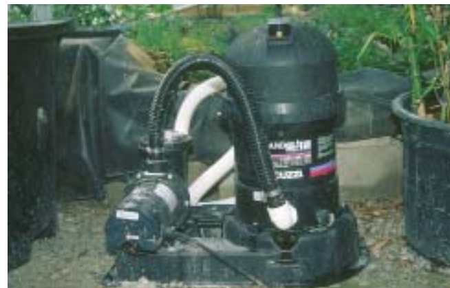
High Pressure Sand Filter
